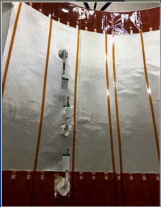
Helium inlet pipe with ground insulation
