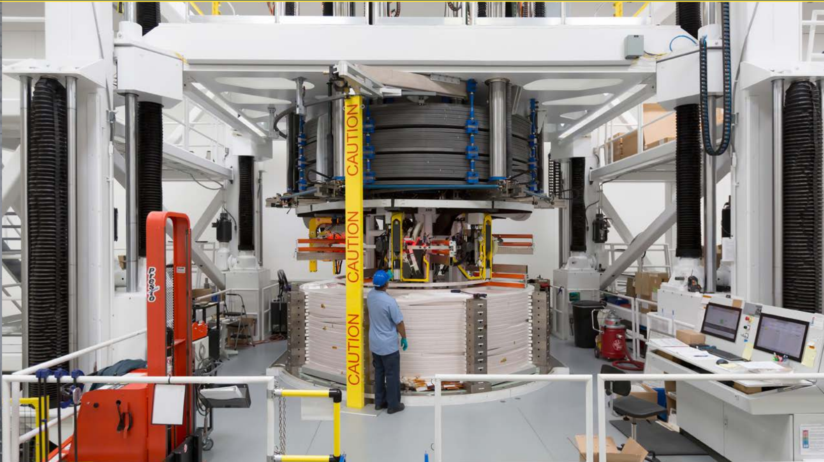
Turn insulation station structure lifts and raises 110-tonne module and releases individual turns for insulation wrapping
