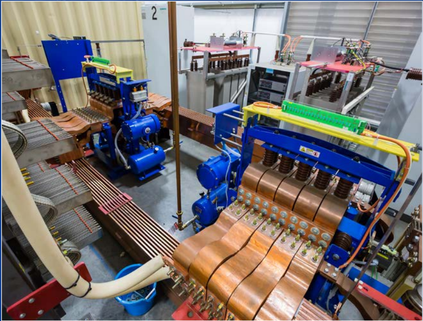
50kA magnet charging power supply with 1GJ fast discharge system including 7kV DC switch and dump resistor for full-current testing of CS modules
